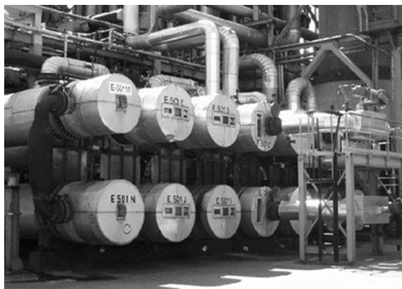
FIGURE 4.13 Photo of Crude Preheat Exchangers
