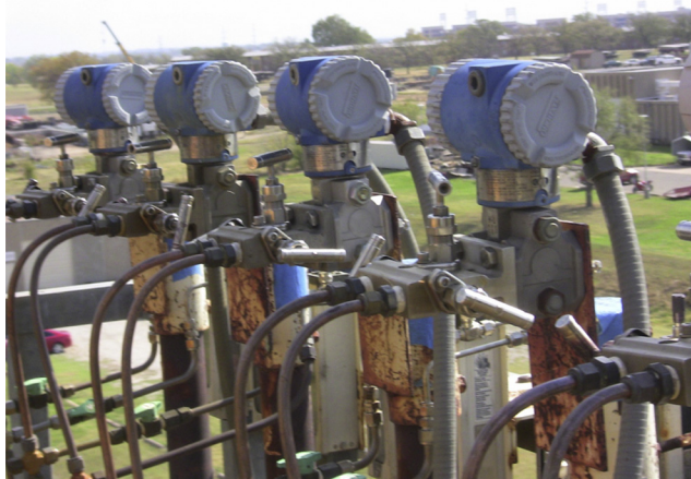
FIGURE 3.14 Differential Pressure Transmitter and Nitrogen Gas Purge Lines
