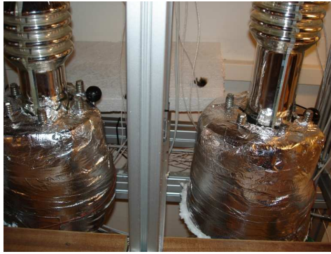
Figure 10.1: First valves installed for the adjustment of the vapor split.
