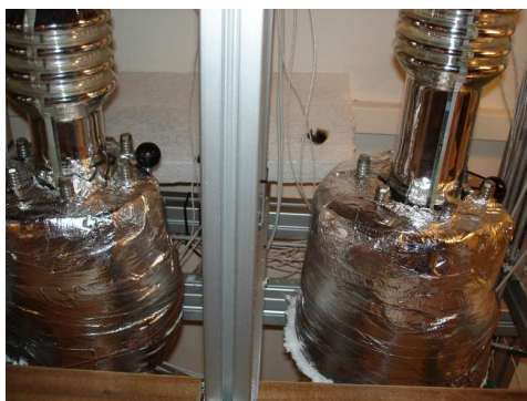
Figure 7.6: Two valves for the adjustment of the vapour split were installed, one on each side of the partition. Here shown under several layers of insulation.
