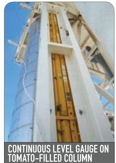
CONTINUOUS LEVEL GAUGE ON TOMATO-FILLED COLUMN Figure 5. During a 100-day processing season, the gamma level gauge remained constant.
