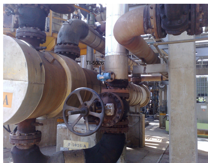
Fig 3. Picture of an installed field device for the second case study 2.
