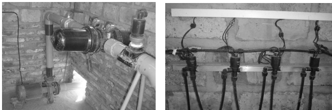
Fig 2: Irrigation head: Pump, filter and electric control valves
