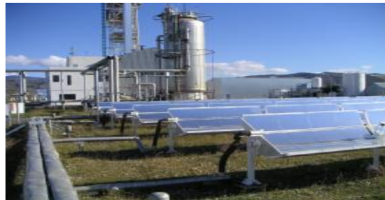
Fig. 1. Loops, pipes and tank of the ACUREX field
