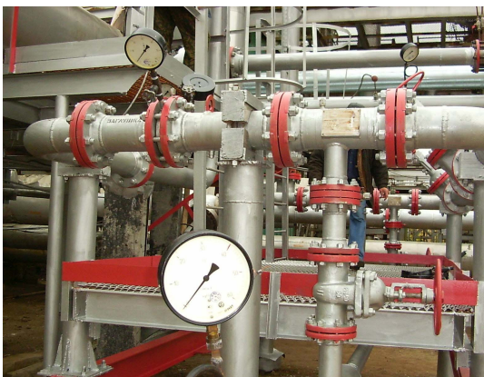
Figure 6: General view of the 3S-facility in Western Siberia
