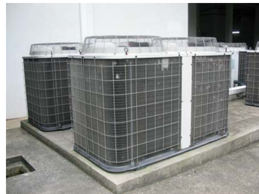
Figure 2 Outdoor unit of PAC
