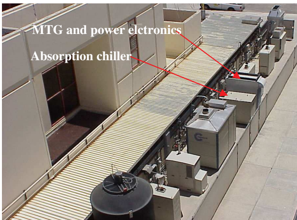
Figure 1: IES unit installed in APEP's test facilities (4 th and 5 th units starting from bottom to top of picture).
