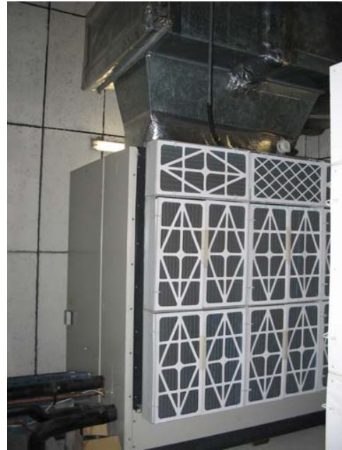
Figure 1 Indoor unit of PAC
