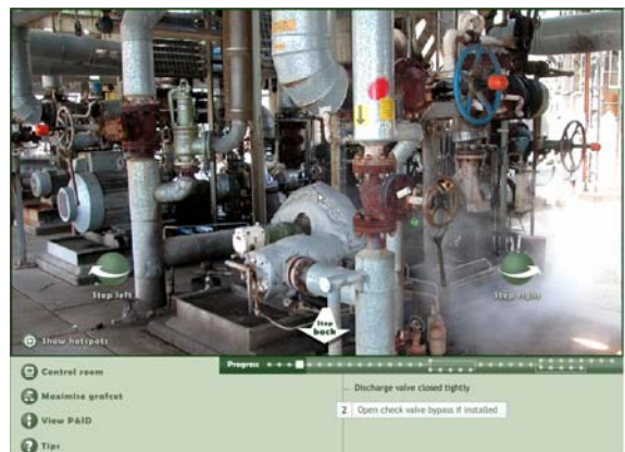
Figure 2 Pump isolation learning exercise
