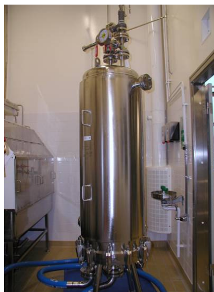
Figure 2: Large scale PALL filter housing
