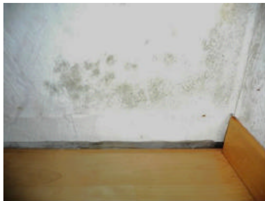
Fig 2. Same corner, no mildew under the baseboard!
