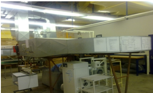
Figure 6 Air Handling Unit (AHU) of UTS laboratory
