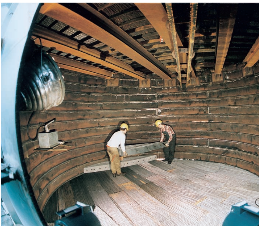
◀ Installation of Montz-Pak Type B1-300 into a column DN 5600 from which the existing valve trays have been previously removed. All supporting rings have been removed by torch-cutting.
