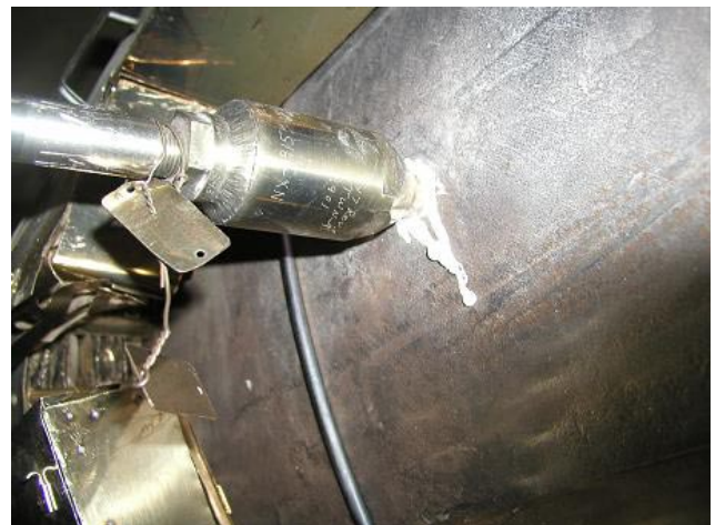
Figure 1. Hot leg instrumentation nozzle with boric acid deposit.
