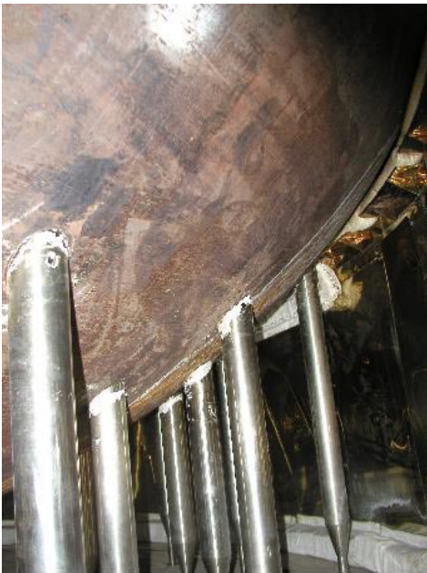
Figure 3. White paint on BMI penetrations
