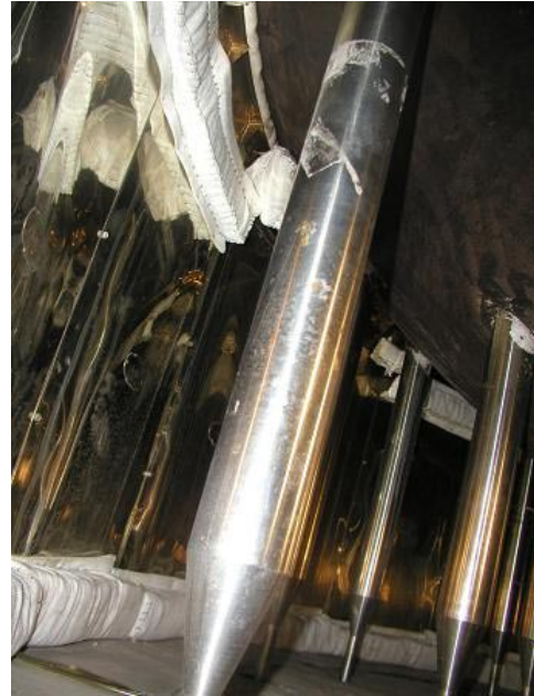
Figure 4. Duct tape residue
