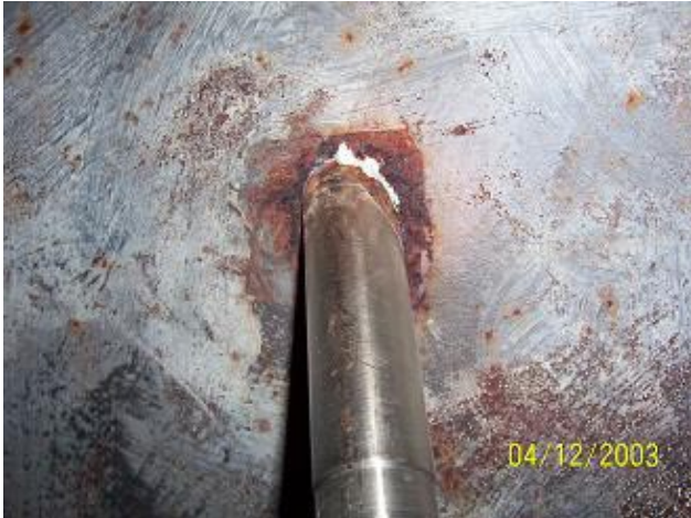
Figure 2. Reactor vessel bottom mounted instrumentation nozzle.
