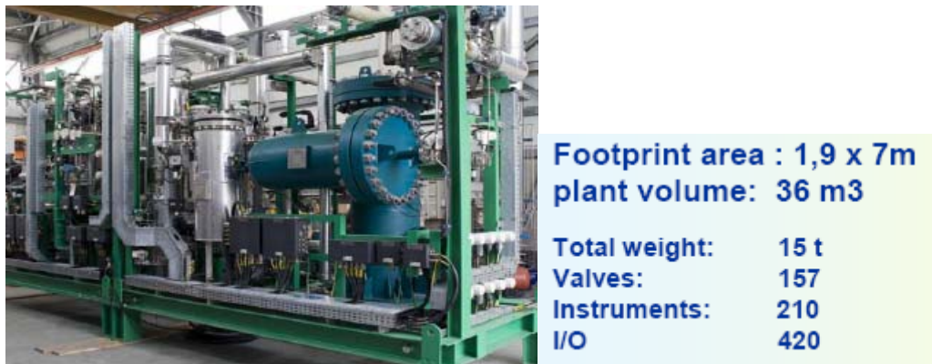
Figure 4. Image of the Air blown SCT-CPO plant located in multi-fuel station in the municipality of Mantova distributing H 2 to FCV and NG, gasoline and Diesel to ICE within the framework of the ZeroRegio project sustained by the European Union ( www.zeroregio.com ).
