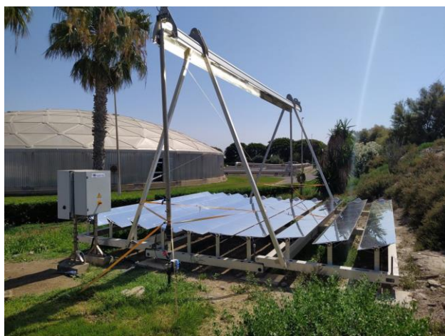
Fig. 1. Demonstration plant based on Fresnel-type solar concentration technology ( El Bobar WWTP, Almería, Spain).
