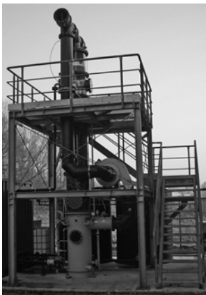
Figure 1: Picture of DN600 test plant for ERA with random packings.
