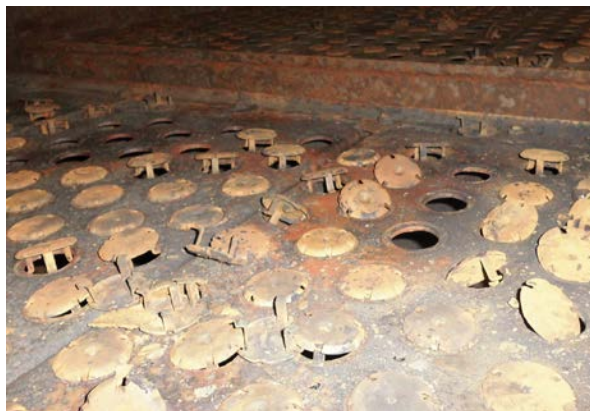
Fig. 5b: V1-valve tray with lost and stuck valves
