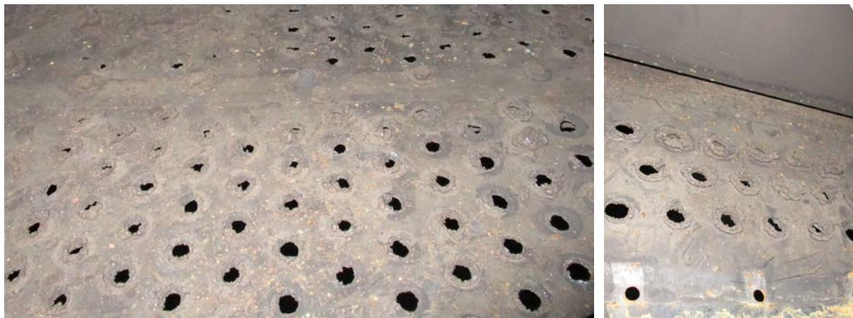
Fig. 2 Crystallization fouling in a sieve tray tower
