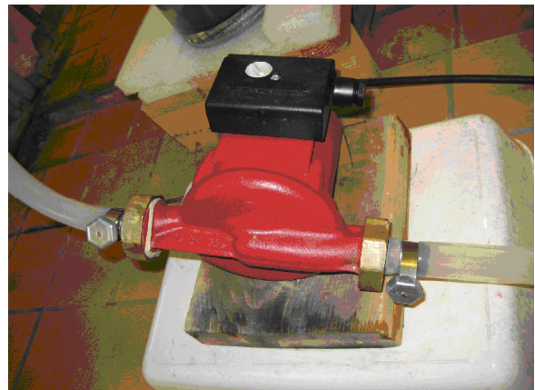
Figure 3.2 The water circulation pump.
