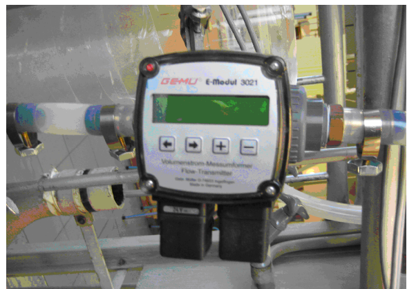
Figure 3.3 Flow rate meter, water.
