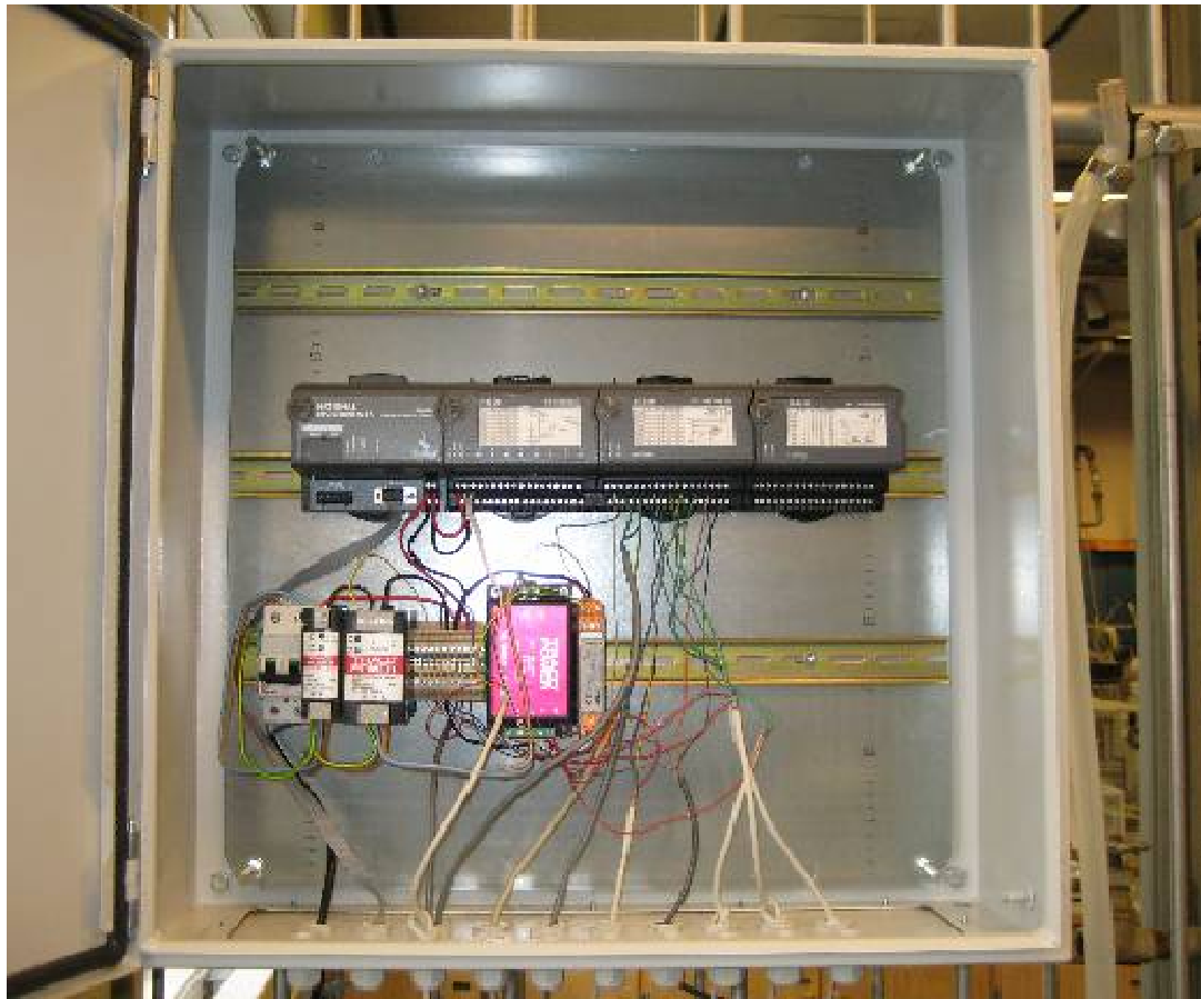
Figure 3.12 The water proof cabinet with the FieldPoint modules in it.
