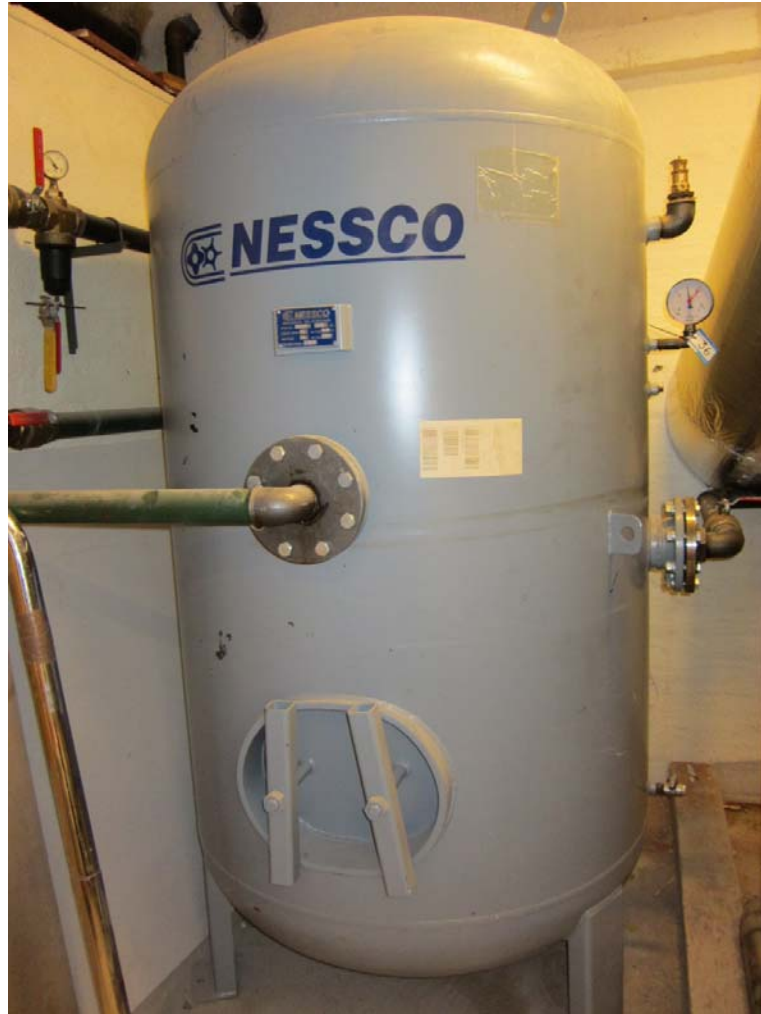
Figure 3.6: Air reservoir tank located in basement
