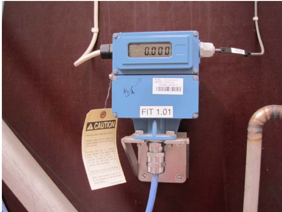
Figure 3.11: Air flow meter
