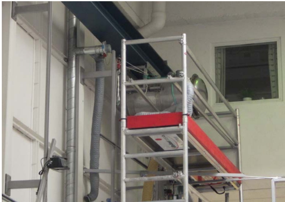
Figure 3.8: Over flow tank at top of riser
