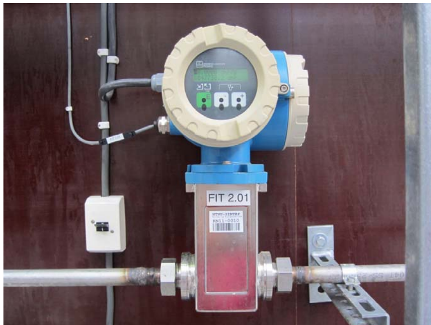
Figure 3.12: Water flow meter
